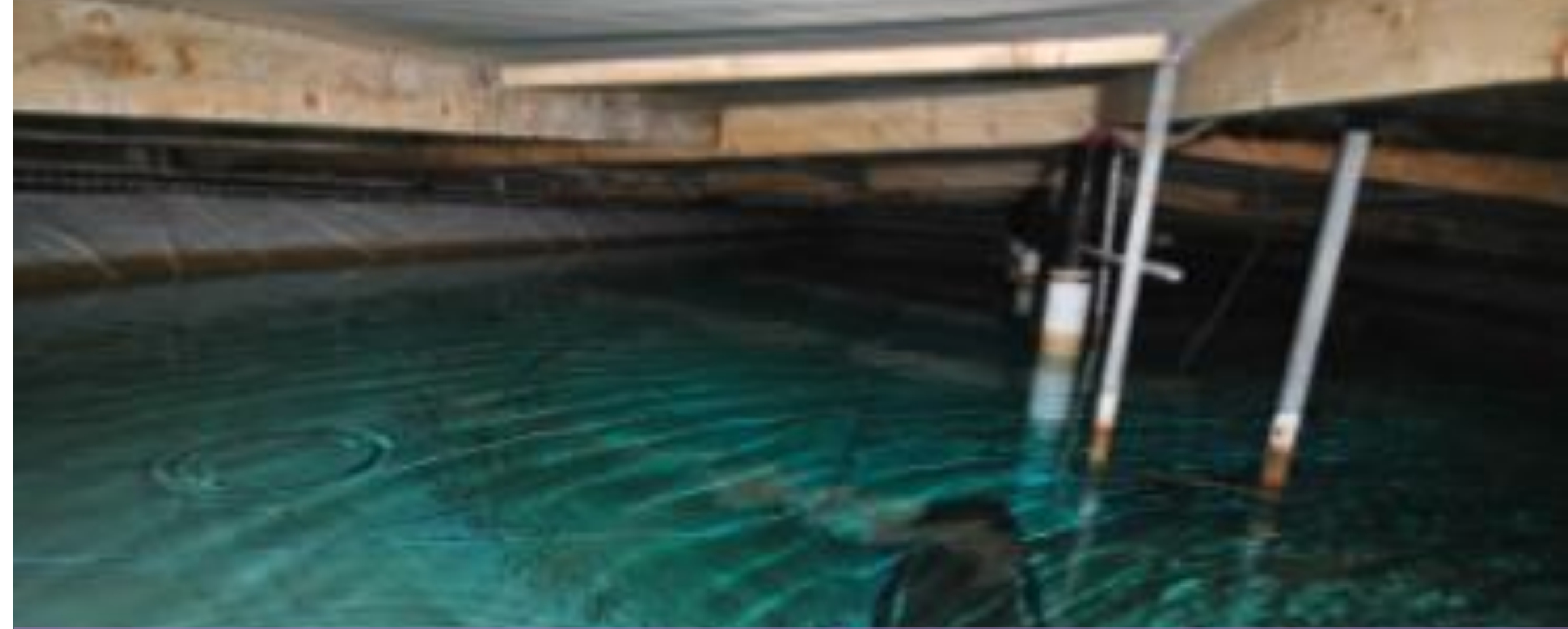
La Jolla Country Club Pump Station & Reservoir Replacement – City of San Diego
